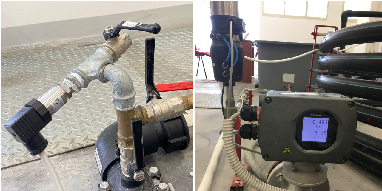
Figure 2. (Left): Pressure transducer installed in a node of the LIA water distribution network. (Right): Electromagnetic flow meter.
